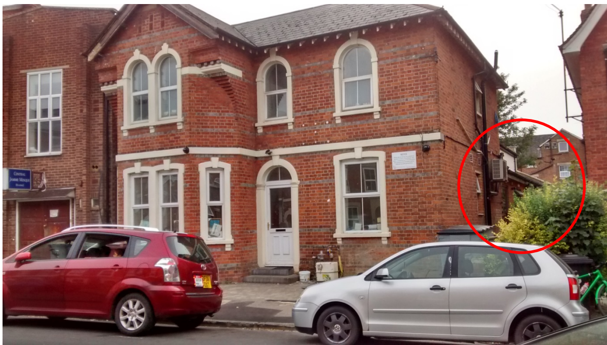
Site in current view from Waylen Street. Unauthorised extension is just visible in the red circle. Front boundary wall is missing.
